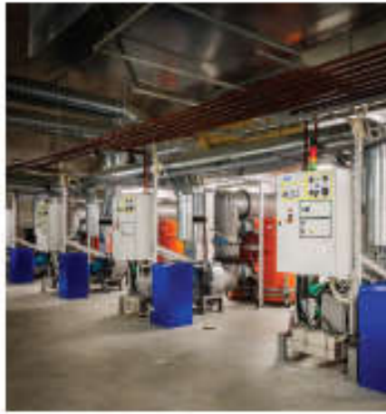
CBRN Filtration units
