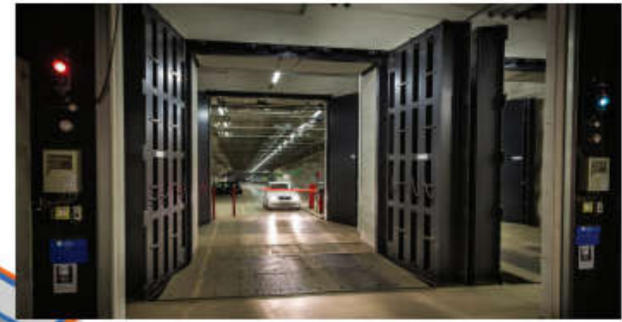
Double Leaf Blast Doors at the entrance of an underground car park
